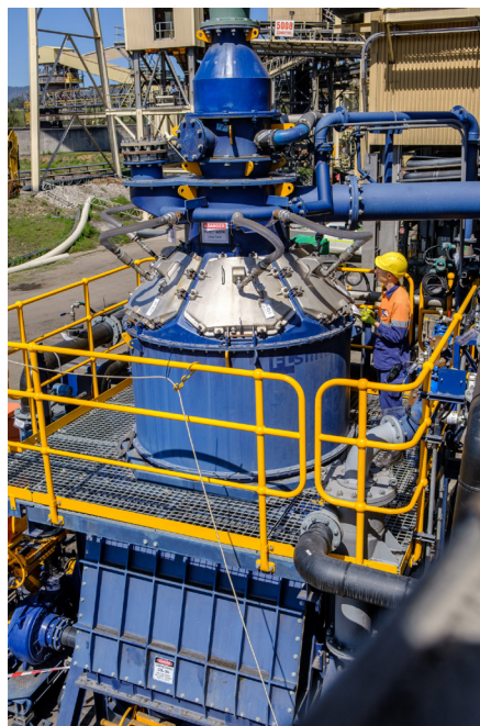
The FLS RFC is now seeing increased interest across metal sulphides and industrial minerals - this shows a full sized cell trialled at KGHM's copper operations in Poland
